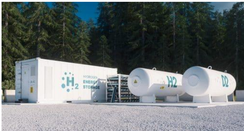
Figure 2.4: Hydrogen Storage, Source: [4]
